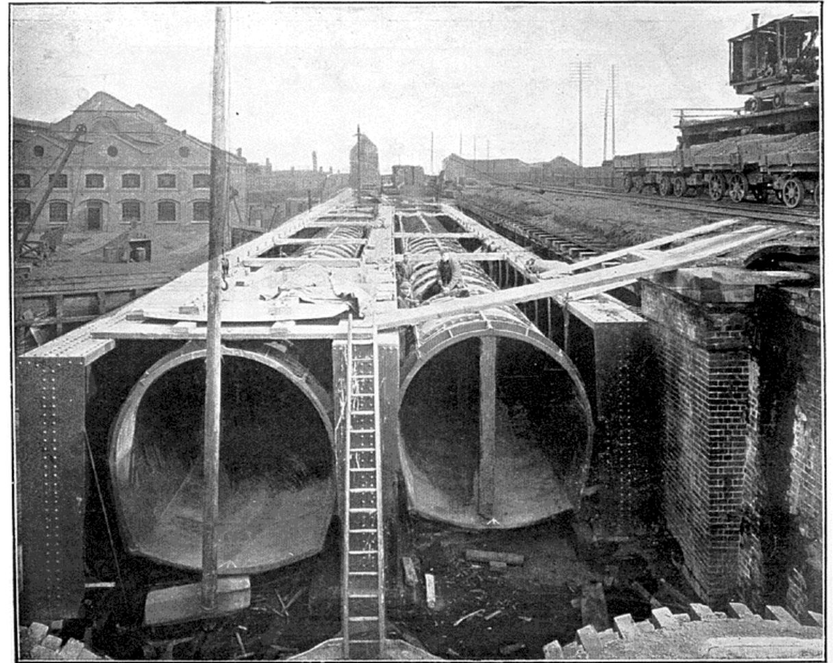
NORTHERN OUTFALL SEWER IN COURSE OF CONSTRUCTION, SHOWING CAST-IRON SEWERS OVER ABBEY CREEK AND CHANNELSEA RIVER. 1902-06.
